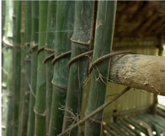
FIGURE 2. Bamboo stems being tied closely in both horizontal and vertical manner for better strength and stability of the bamboo hut.
